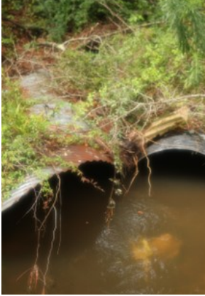
Drainage ditch that no longer functions and needs to be upgraded
