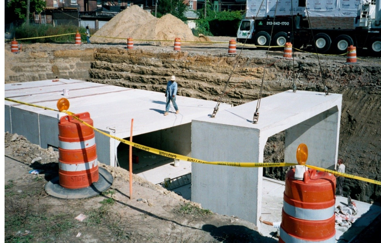
Vault / Underground Storage
