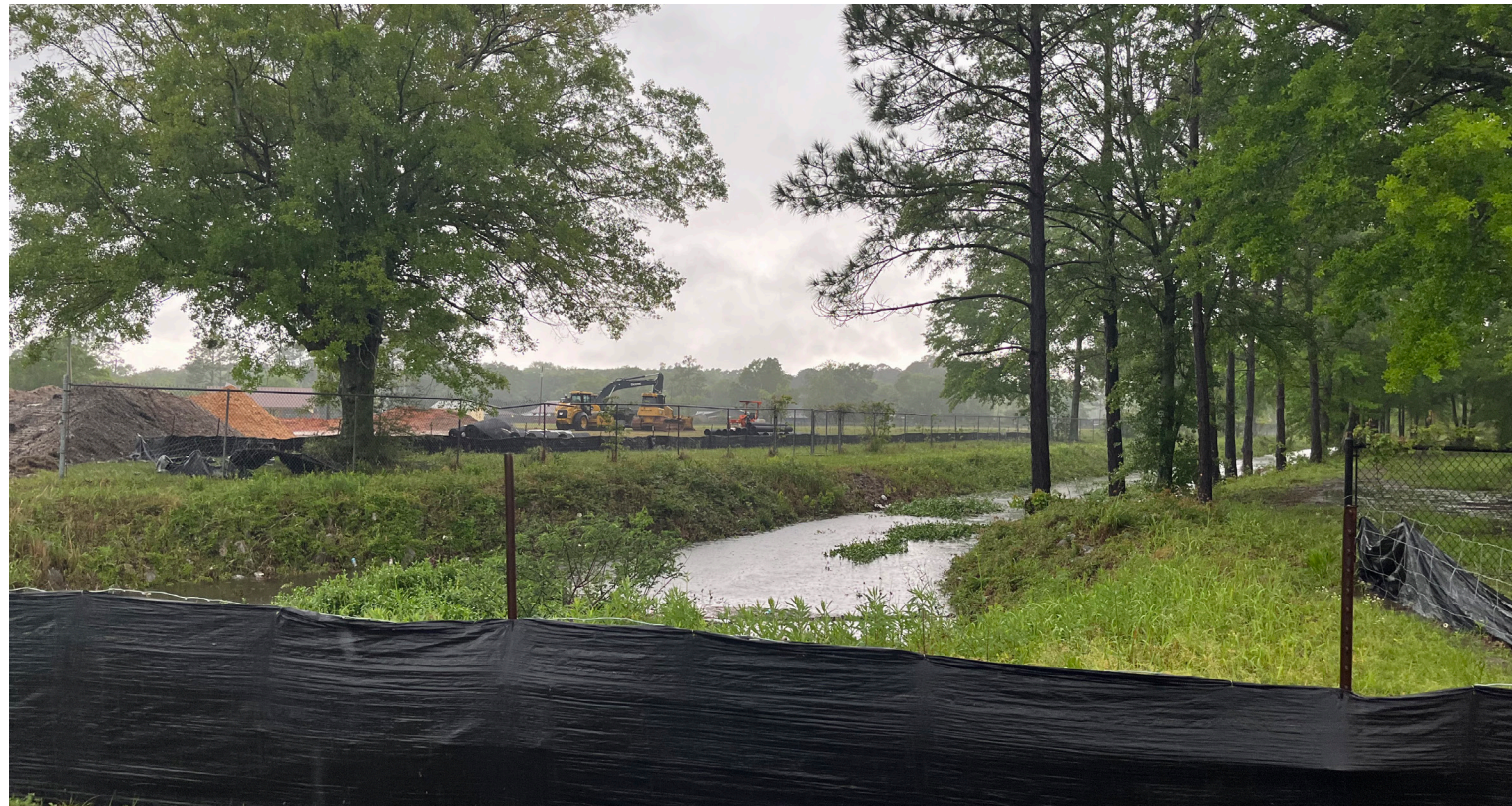
3 | Construction of New Parking Lot at Khayat Park, Looking West from 2nd Street
