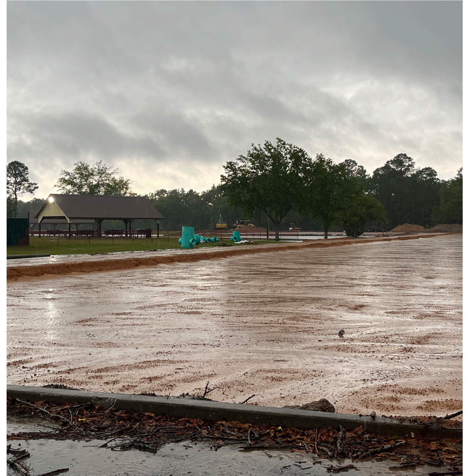
As of April 10, 2024 the eastern portion of the site was under construction for additional parking in Khayat Park, see IV Appendix - iv.
